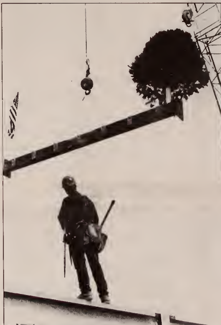
Going up . . . A worker watches as a glider bearing the American flag and an evergreen tree is hoisted into the air to be placed at the top of a building in the University's Research Park as part of the topping-off ceremony held on April 14.
